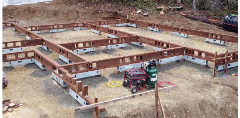
16. Construct the cripple walls on top of the sill plates per the plan. Frame cripple walls off the sill plates to specified dimensions.
