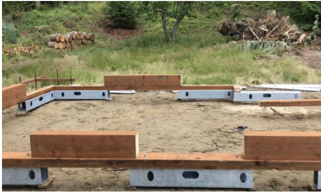
15. Continue installing the sill plates and headers. Ensure end cuts are treated.
