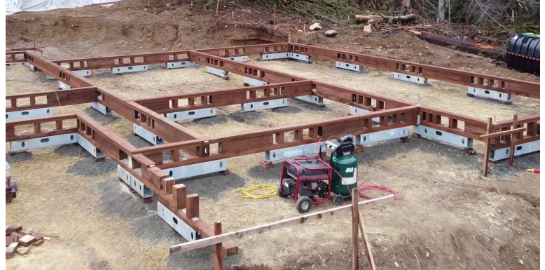
16. Construct the pony walls on top of the sill plates using 2"x 6" crippers as per the dimensioned plan. Frame pony walls off the sill plates to specified dimensions.
